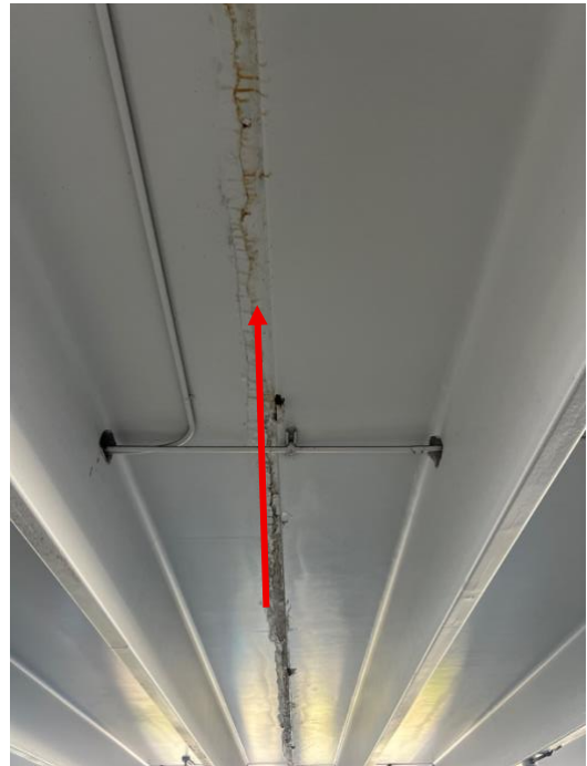
No lead detected in white concrete ceiling joint paint inside the International Parking Garage
