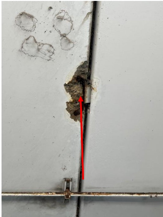
No asbestos detected in spalled concrete ceiling joints
