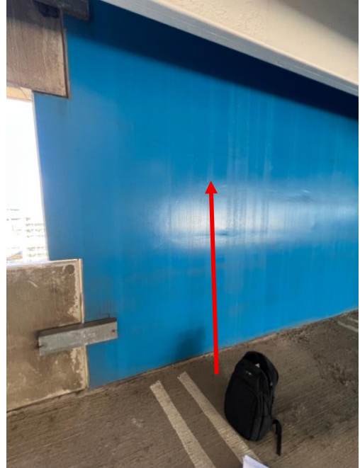
No lead detected in blue wall paint inside the International Parking Garage
